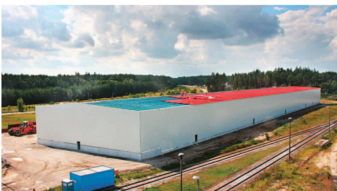
The construction of the pipe and spare part warehouse began in April this year and was completed in August.
